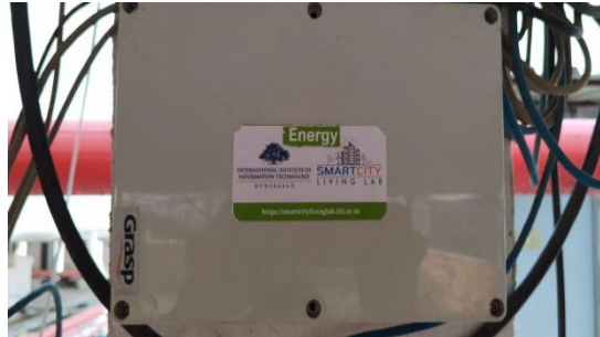
Figure 23: Smart Room Energy Monitoring
