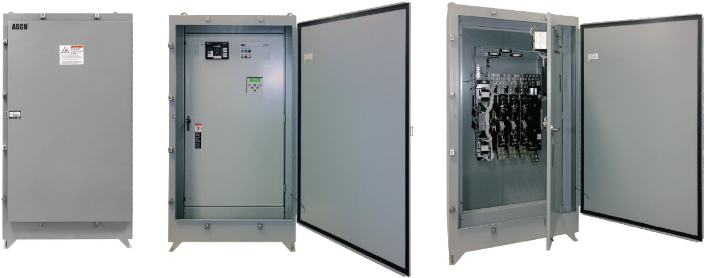
Figure 8: These views show the double-door construction of a secure Type 3R cabinet. When fully closed and secured, the controls are protected from unauthorized access.
