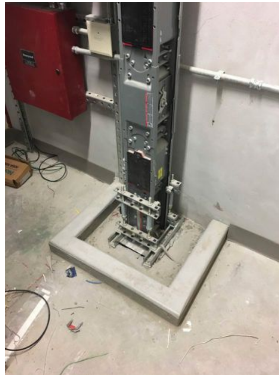
Figure 3: This is a vertical section of busway (or busduct) with no plug-on devices. The waterproof curb is visible in the bottom of the photo showing engineering supports bracing against the floor spanning the entire penetration. This has been sealed with intumescent material below the cover plate for fire protection between floors. Courtesy: NV5
