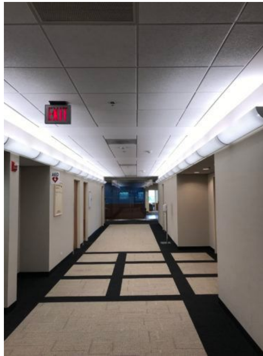
Figure 11: Picture of an older incandescent exit sign where the sign is unusually dim and the direction chevron is difficult to see. Exit signs must have enough visual contrast from the surrounding environment to allow quick identification.
