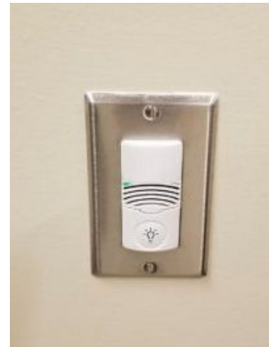
Figure 1: An occupancy sensor with dual technology (passive infrared and ultrasonic) is shown. The button with the light bulb image is pressed as a manual on or off to control the lighting fixtures manually. Courtesy: Metro CD Engineering
