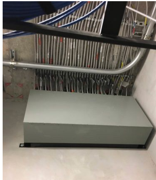
Figure 1: This is a gutter installed in a high-rise building that is provided as an accessible splice point. The level above is the serving electrical room and there are sections of EMT that connect into the top of the gutter. Within the gutter the contractor has spliced, via wire nuts, to connect to the horizontal runs of MC to horizontally feed the guestrooms. Courtesy: NV5
