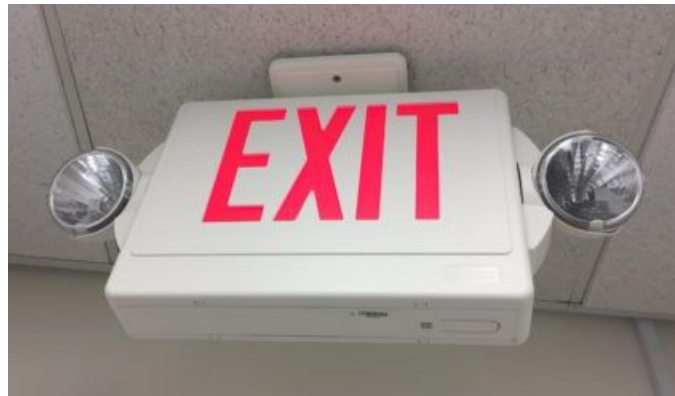
Figure 9: Lamps for emergency illumination are often integrated into exit signs to reduce installation cost. The lamps need to be aimed to avoid blinding people who are walking toward the sign.
