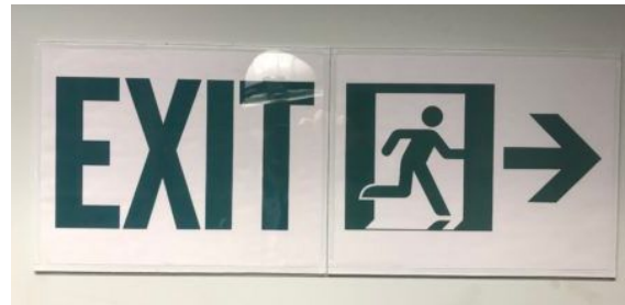
Figure 2: Exit signage using a pictograph compliant with international ISO standard and NFPA 170-2018. All graphics courtesy: McGuire Engineers Inc.
