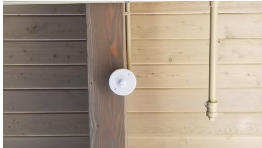
Figure 2: A daylight harvest sensor is mounted on the ceiling in an open multispace room. This sensor will automatically dim the LED lighting in this space based upon ambient daylight. Courtesy: Metro CD Engineering LLC
