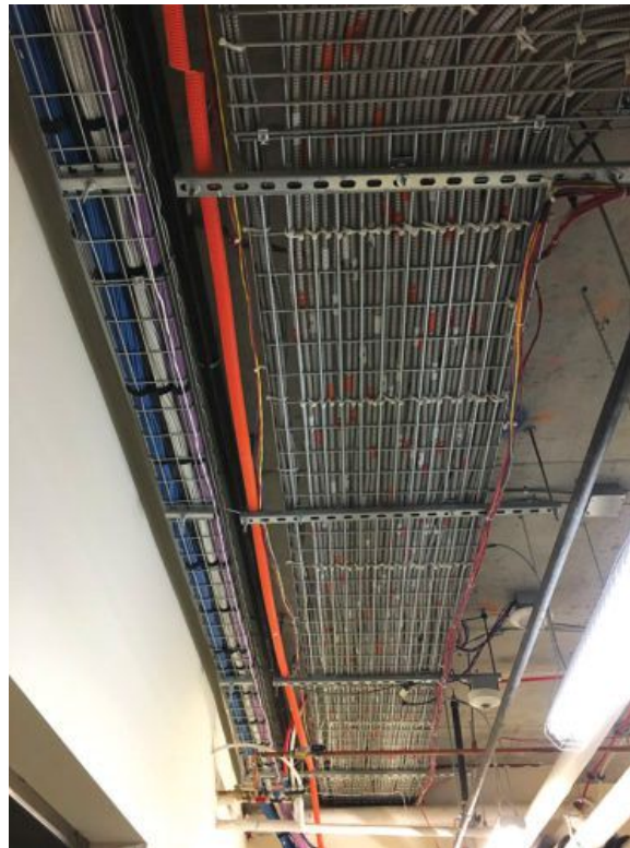
Figure 4: On the right, cable tray is used to support and secure MC wiring as a main routing point down the corridor. In the center, there is an orange innerduct that is used for fiber routing and on the left, there is a cable tray with cleanly segregated low-voltage cabling. Courtesy: NV5
