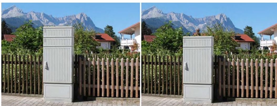
Figure 15: Outdoor cabinet with spatial infrastructure separation for multiple operators
