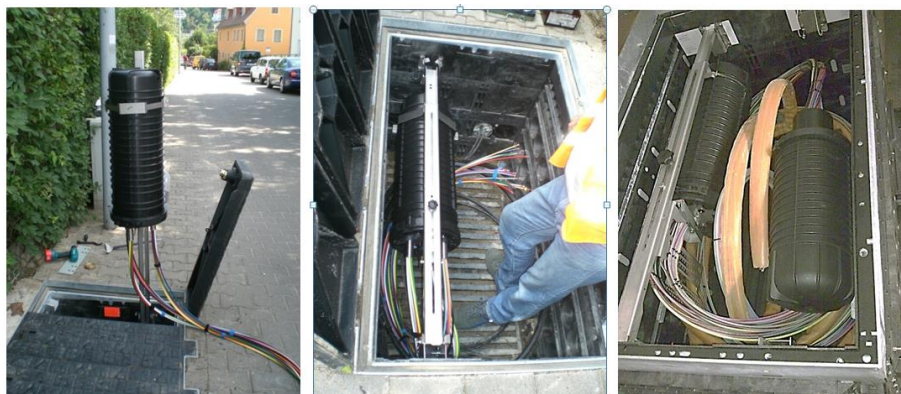
Figure 13: Underground fibre distribution with closures
