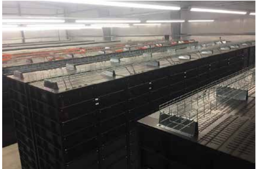
Festival Hydro battery storage facility.
