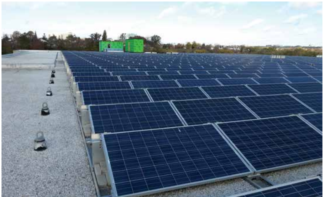
Commercial rooftop solar array.
