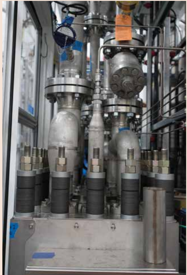
Electrolyser at the Enbridge Power to Gas facility in Markham, Ontario.
