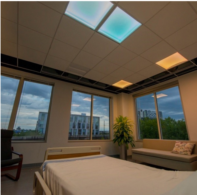
An LED patient room lighting system.
