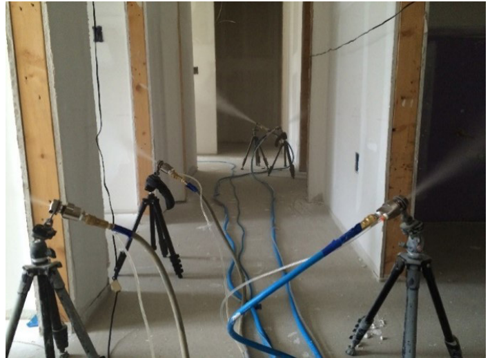
Field testing aerosol envelope sealing in new residential construction. Image courtesy of Center for Energy and Environment.
