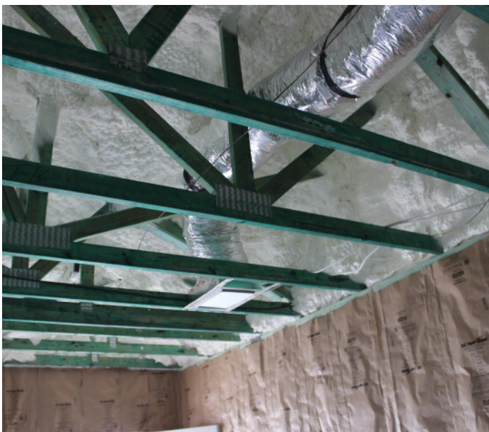
Spray foam insulation provides a conditioned attic space for heating and cooling ducts. Image courtesy of Habitat for Humanity South Sarasota.
