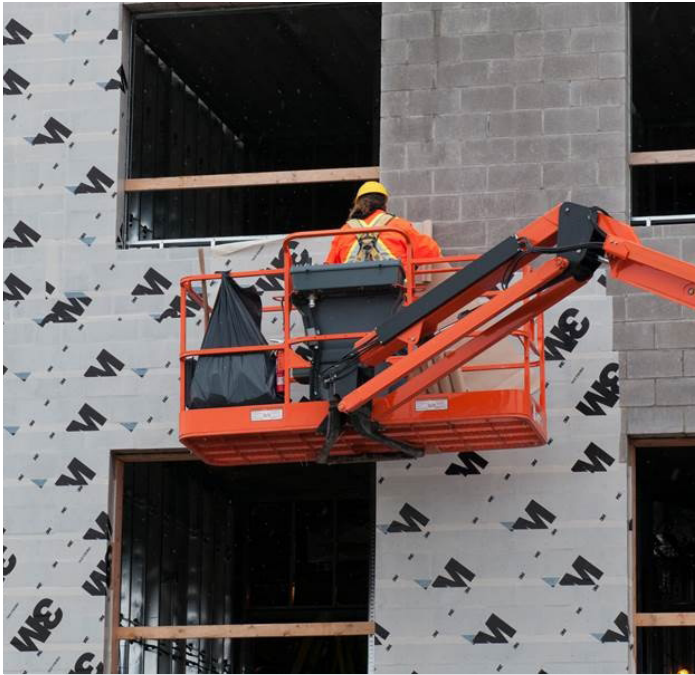
Installation of a primer-less self-adhere membrane that serves as an air, liquid water, and water vapor barrier. Image courtesy of 3M.
